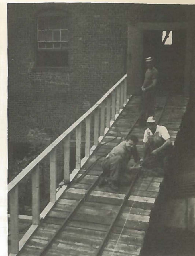
ALLAN DEYO, BILL HOYT and GEORGE BOYER are shown laying rails on the rebuilt pig iron ramp.
