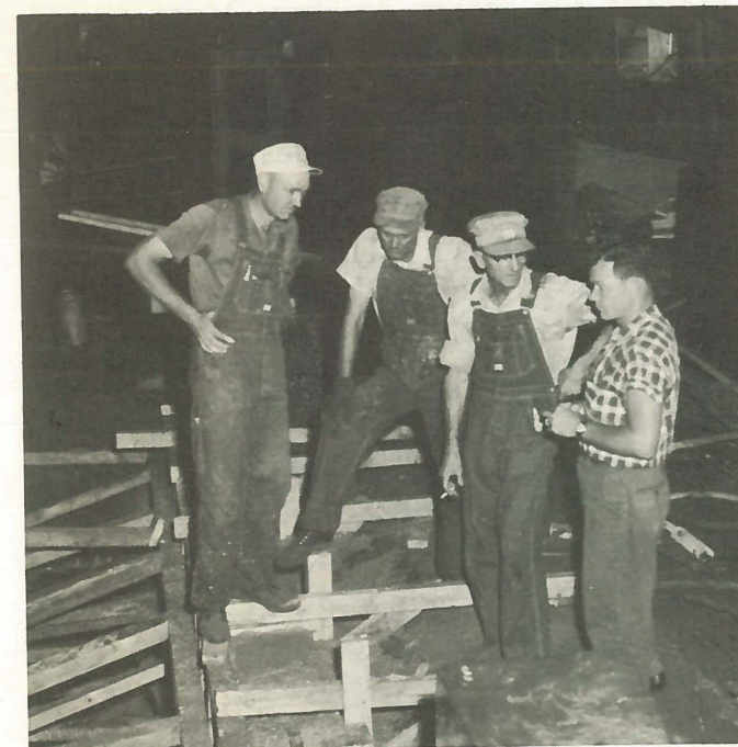
"Four heads are better than one". Left to right, Junior Wilcutt, Carpenter; John Jackson, Crane Operator; Jim Hollis, Carpenter; and Bill McCain, Engineer, discuss form building for concrete wall.
