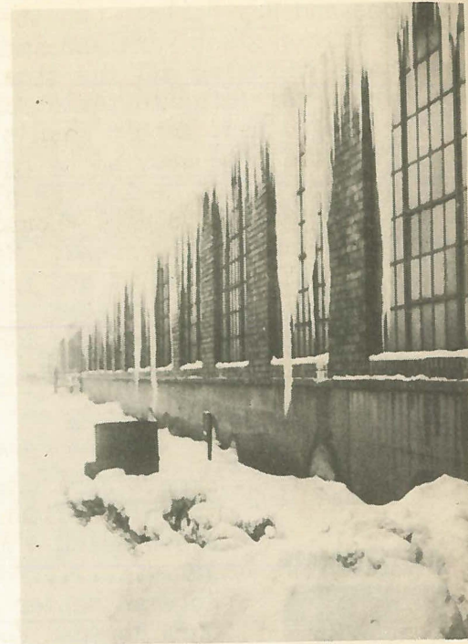
Some of the giant icicles on the Gasteam Assembly Building.
