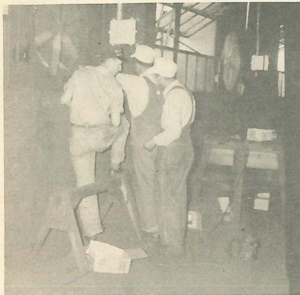
James Layton, Ewen Self and T. J. Williams are installing additional fans in the deLavaud Foundry.
