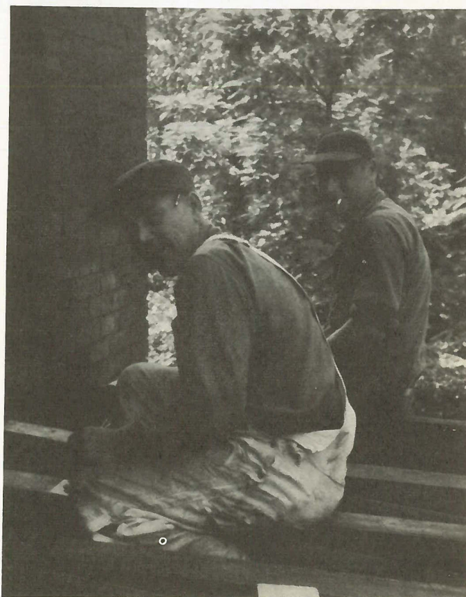
Carpenters BILL HOYT and MARIO CUCCHI prepare a level base for the platform floor.
