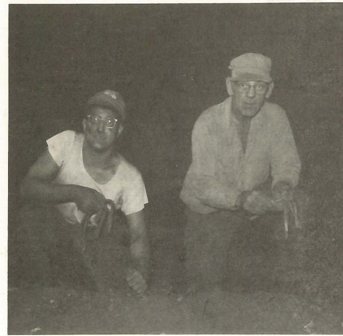
VINCE MASTROPIETRO and TOM NAPPLES in the process of cleaning up the molding floor. Forms for the concrete floor will follow.
