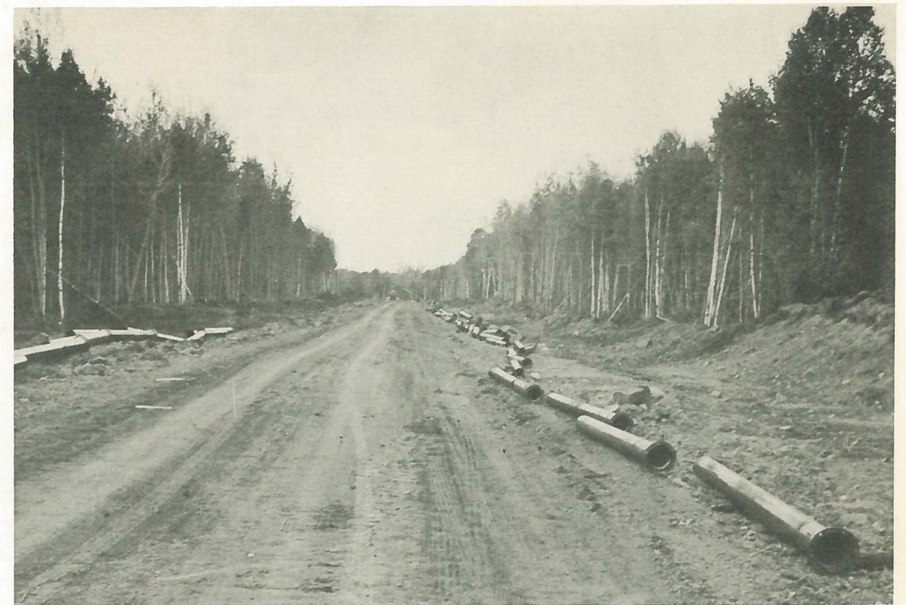
Lengths of Clow cast iron pipe that will carry water to the new homes at Beaver Bay, Minnesota.
