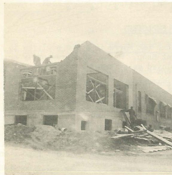
At left: The new office extension for the Engineering section is progressing very well.
