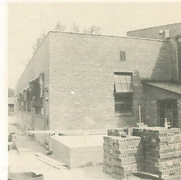
Above- The floor has been poured for the new First Aid and Personnel office
