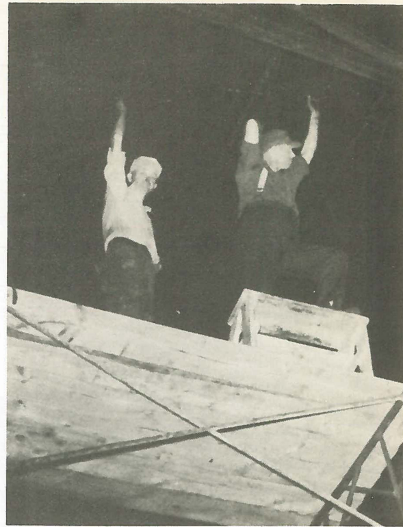
Installing the sprinkler system in the Ream & Test Department, Cecil Gardner (light shirt) and Glenn Shaw.
