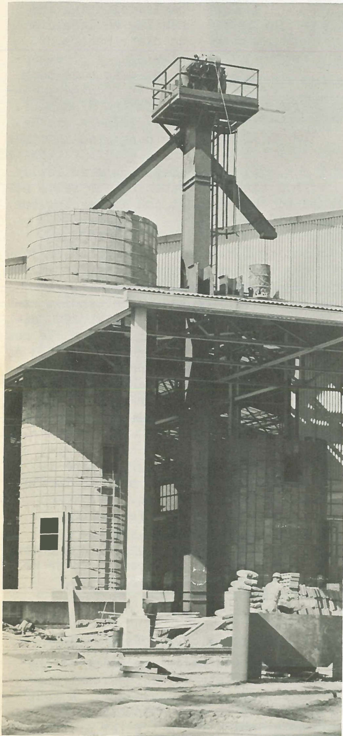
View shows the two socket core sand silos and sand unloader at the South end of the Pipe Shop. Silo at left is at full height.
