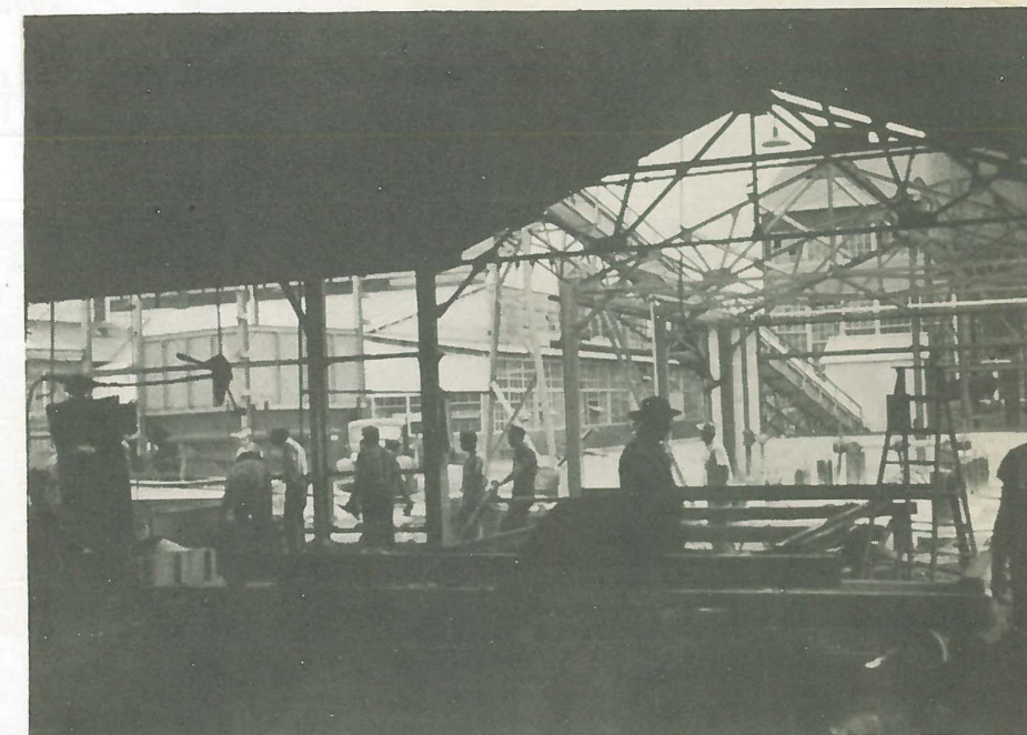
Here is a view of the construction work on the cement lining department.
