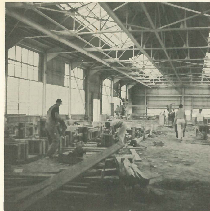
View looking west, down the Pipe Finishing Run, showing construction work underway in building the Tar Tank in which pipe are coated after cleaning, before shipment.
