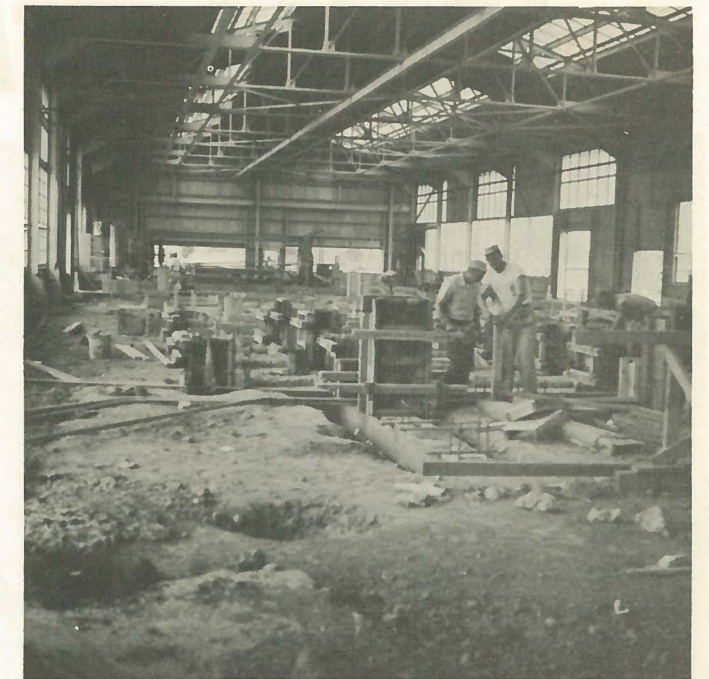
Above, a general view of the Finishing Run, which shows the concrete bases for pipe rail supports, on which pipe are rolled down the run in finishing operations.
