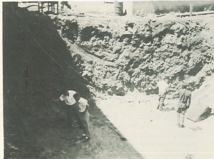
Irvin Goodwin and H. J. Franklin survey the excavation work being done behind the Power House. This project is a part of the new Cement Lining Department.
