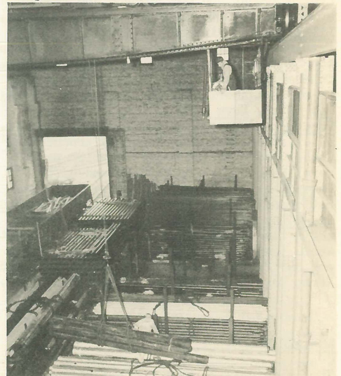
TRAVELLING CRANE can unload a gondola in a matter of minutes. Rope slings on each pipe simplify pickups
