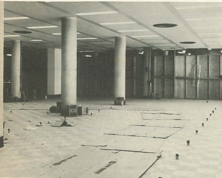
Completed office area above, shows new light fixtures and air conditioning outlets, flush mounted in the new acoustical ceiling. New flooring has been laid and electrical outlets installed.
