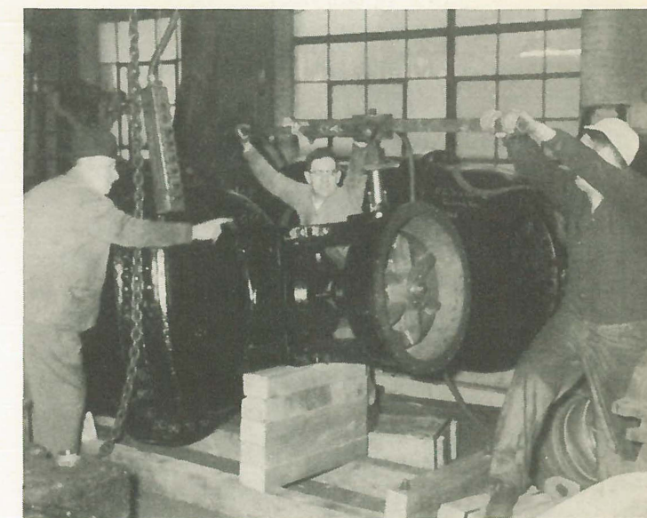
Above: As foreman Frank Galerie directs the operation, Matt Curley and Gerald Lahue run a gate operating test with a motor driven operator.
