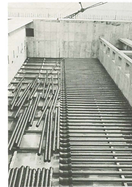
Partial installation of long pipe into Bell-tite joint of tees in one bed.
