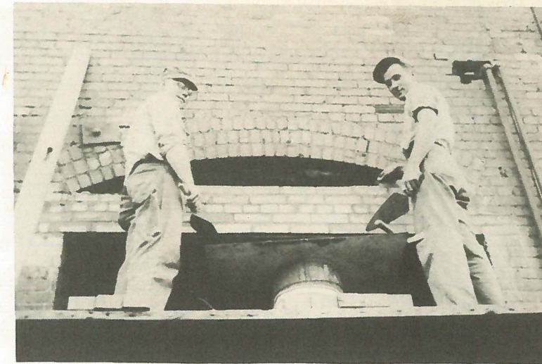
Bob Temple, left and Lester Gadd, have been giving our foundry buildings a little more modern look this summer. They are replacing the old wood frame windows with steel ones.
