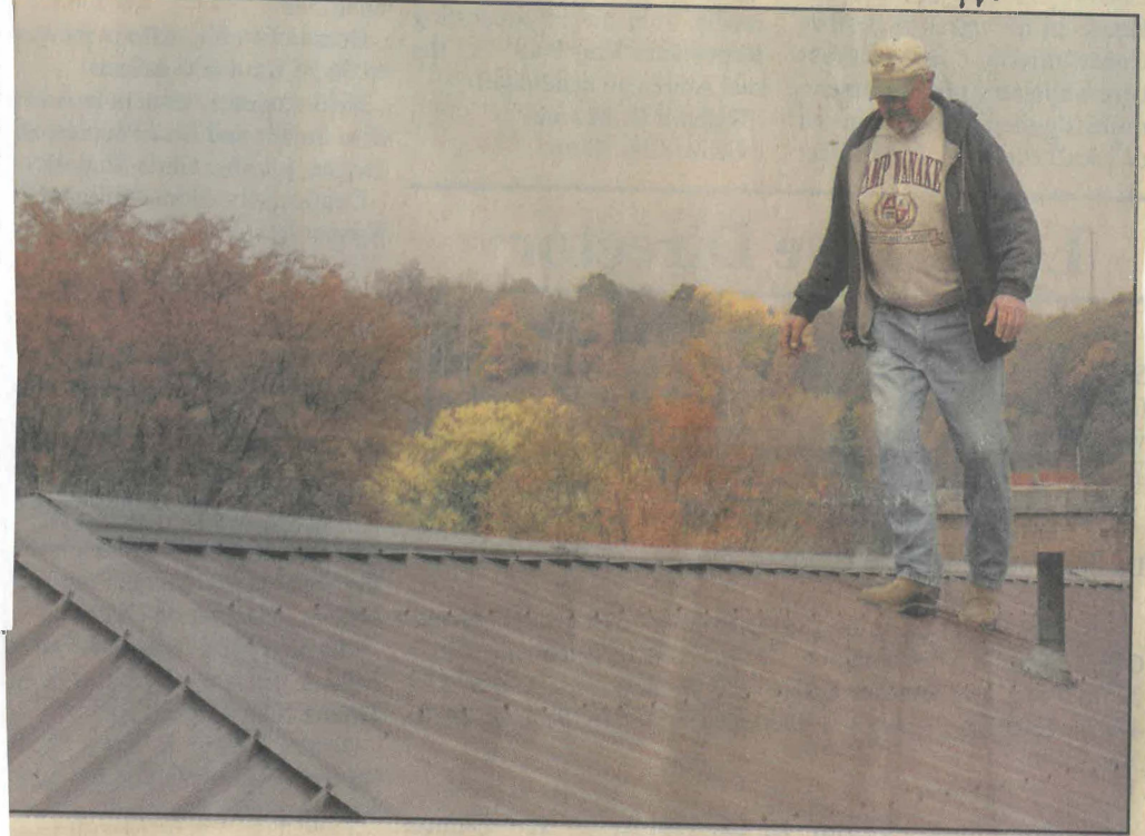
Ray Booth / Newcomerstown News Rick Peterson of Newcomerstown treads carefully along the roof line of Christ United Methodist Church. A group of volunteers continued their work recently to get a new metal roof in place before winter weather hits.
