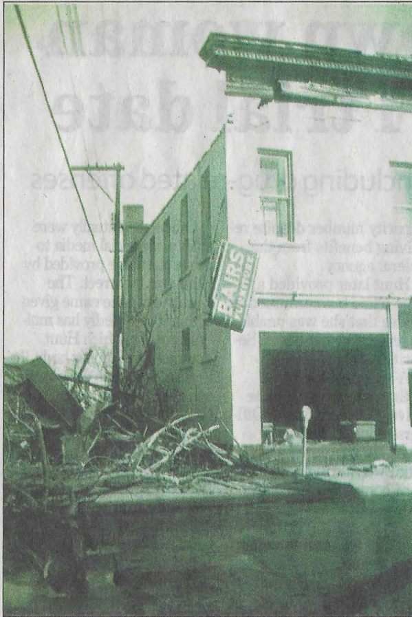
Bair's Furniture on Main Street is seen with substantial damage to the building's roof. The front window was completely shattered, and the alley-way next to the building was obstructed with tree limbs, and debris.
