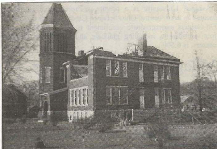
File photo The aftermath of the March 11, 1955, tornado is pictured here as a portion of the East Elementary School roof and top floor of the building was damaged.
