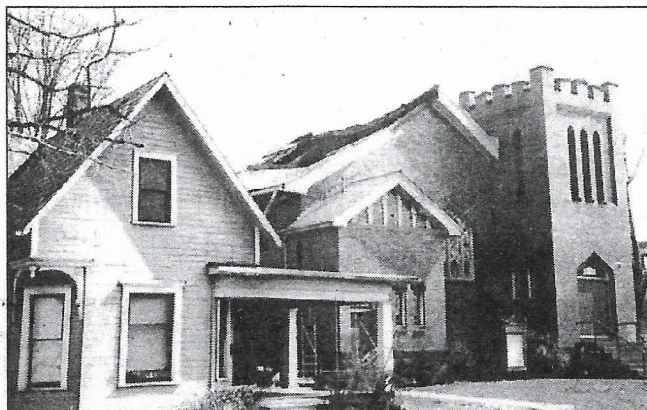
■ The north side of the roof of the St. Paul Evangelical Lutheran Church was damaged, requiring replacement.
