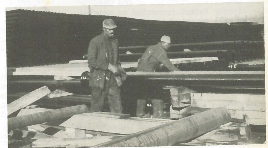
At right - Tom Parker and Ocie Miller are transferring pipe to the storage runs.
