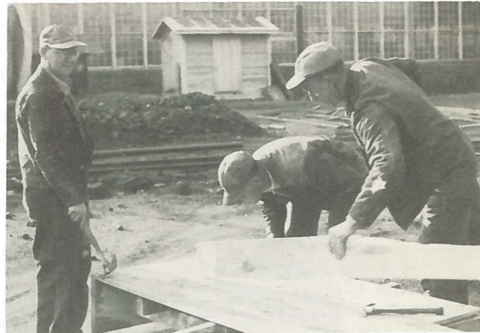
Claude Tittle , H.B. Hannah and Houston Smith are building forms to be used in the construction of the new Cement Lining Department.
