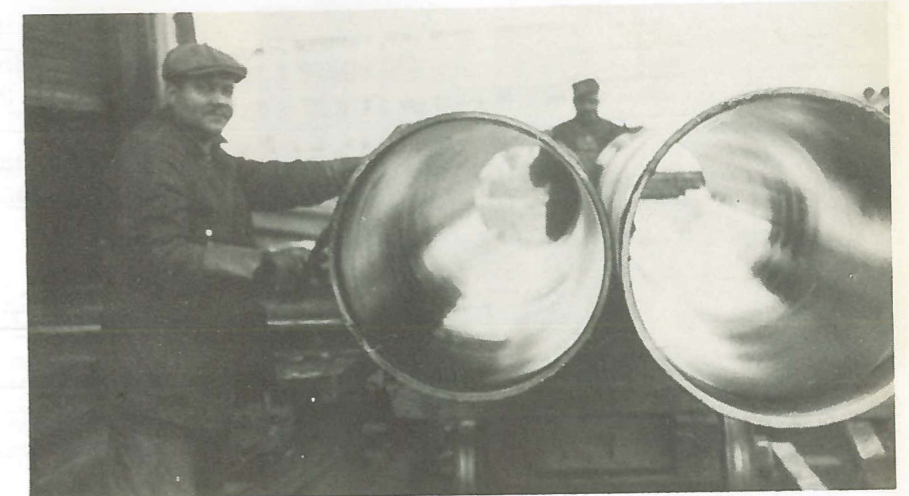
At right - Payton Dunnavant and Walter Cole are touching up pipe as they leave the Cement Lining Department.
