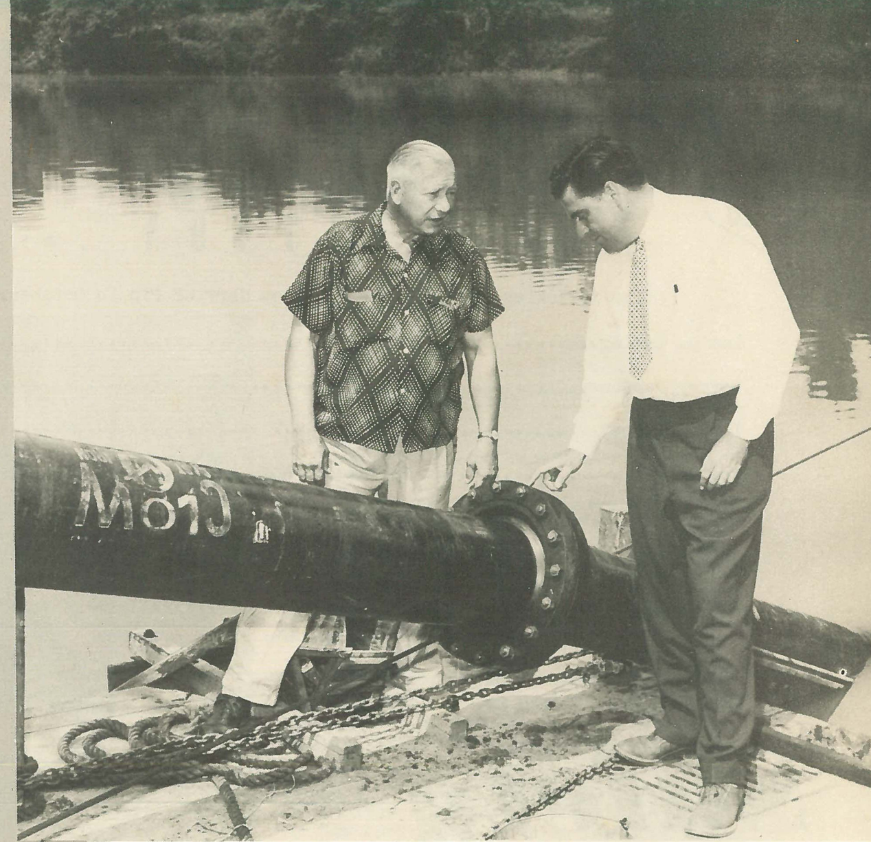
Guil Falcon, left, of the Falcon Marine Company and Ray Rinehart, our Clow Sales Representative who operates out of South Bend, Indiana, look over the installation of the first Clow manufactured River Crossing Pipe at Defiance, Ohio.
