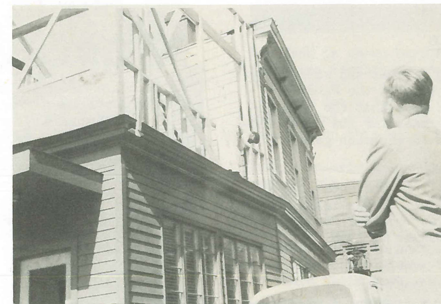
Sales Manager, Bill Weber, views the work being done to expand his Sales Office. Another step forward in the progress and expansion at Eddy Valve.
