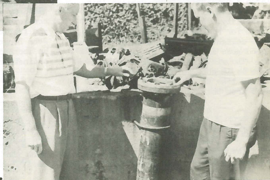
Dick Michaels, left, and Tom Voss are shown examining the broken hydrant flange.
