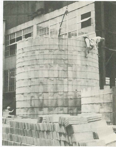
Construction still continues on the new Specials Foundry. Here's a picture of the actual construction on one of the new sand bins.
