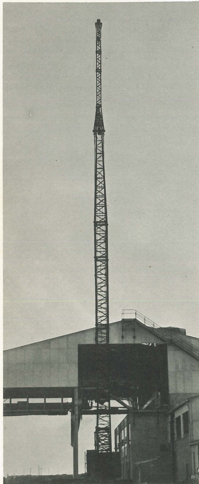
Towering high above the roof line of the Melting Dept. Iron Yard shed is this crane with a 130 foot boom, used to set cupola shell segments in place, and do other otherwise "impossible" construction jobs.
