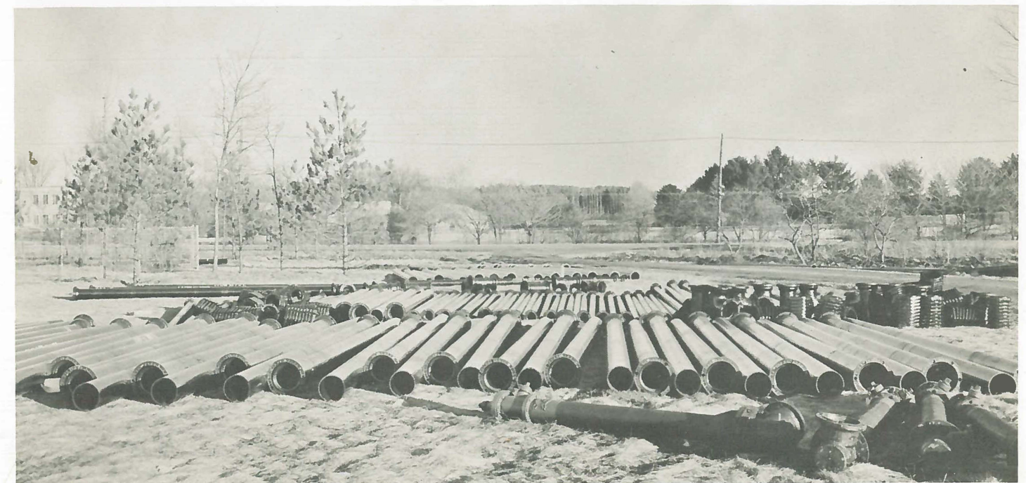
Below is the stock of pipe, fittings, valves and hydrants which were used on this installation at the Morton Arboretum.
