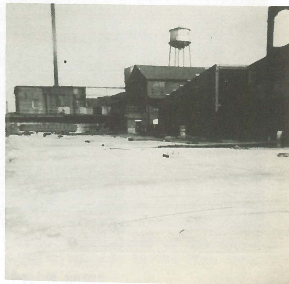
At right: New concrete floor for the extension on the north end of the Pipe Foundry.
