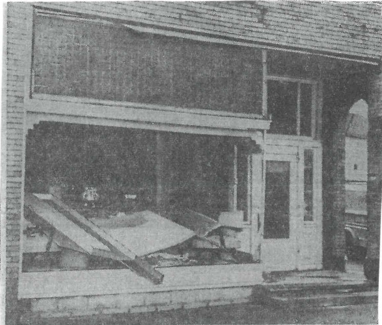
The display windows and the front were caved in at Cooper's furniture store on West Main st.
