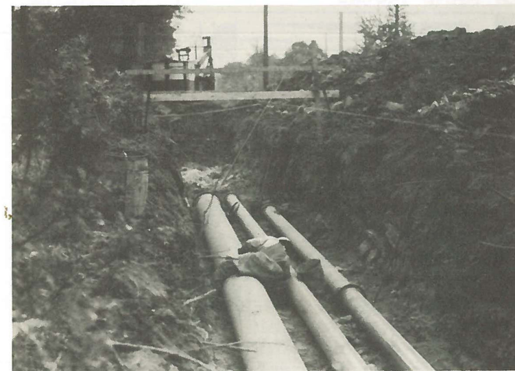
National will have a new neighbor. Work has already begun on the Ketona Chemical Corporation whose property is close to National. Plans call for the plant to be in operation by early 1956. Of course, we are glad that our new neighbors are using Clow pipe and this is a view of the installation of some of our product.
