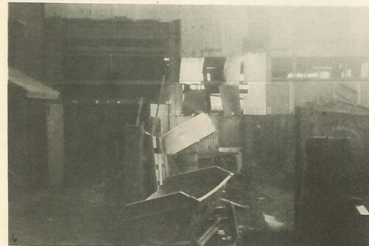
Our shot of the north wall wasn't too good for we had the sun in our face. This wall was nearest the cupola and the one that suffered the most damage.
