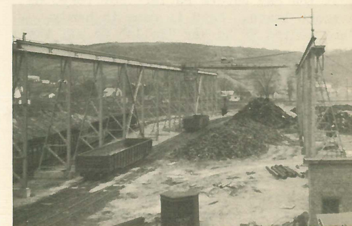
Showing the new Industrial storage crane in action.
