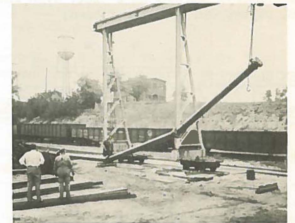
River Crossing pipe with a deflection of 15° on two sections under pressure.
