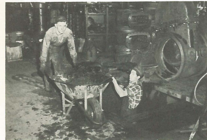
Keith Ward, left, and Don Allgood are busy doing a maintenance job which can only be done when the plant is not operating. Here they are cleaning sludge from the large valve mounting pit.
