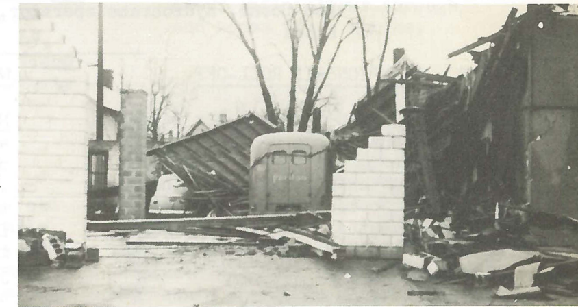
Service garage demolished by tornado. The 1948 Ford on the left belongs to Mrs. Mary Kitchen .
