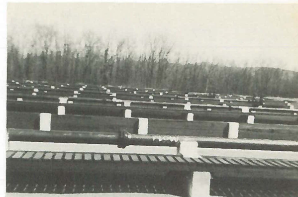
Clow pipe used in Sewage Disposal Plant at Coshocton, Ohio.
