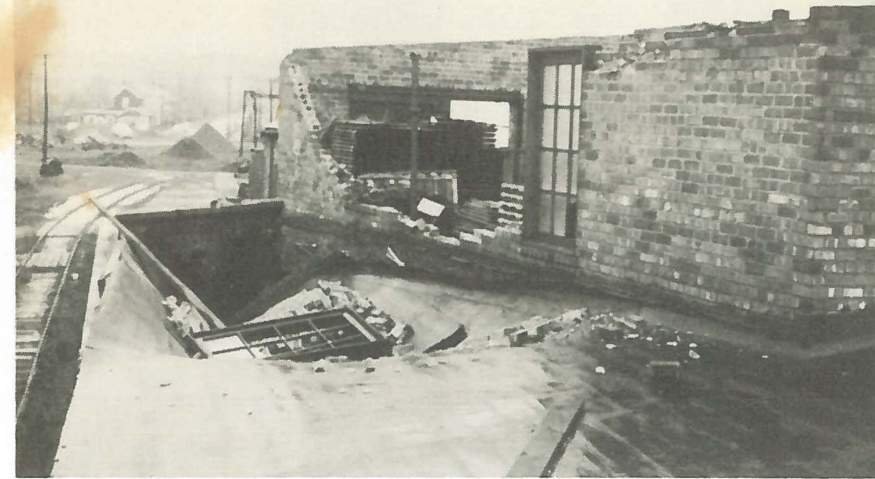
The roof of our unit heater storage building was blown off and the east side of the brick building was blown onto and through the roof of the adjoining building.
