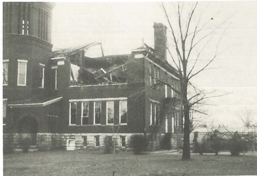
East Elementary School building was badly damaged by tornado.
