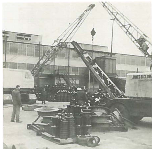
Removing the last of the old bridge crane in the Shipping Yard.
