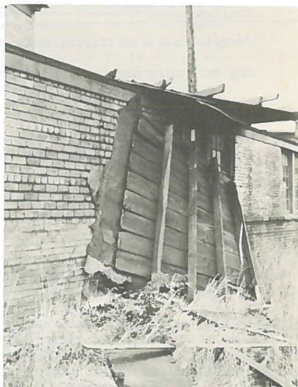
Portion of the roof was blown into the yard.
