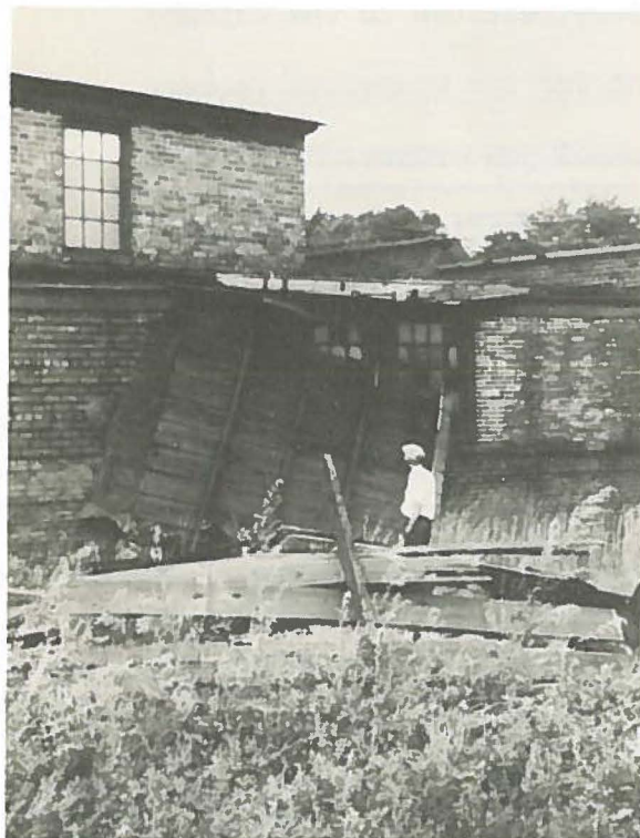
Elmer Wise, Maintenance Foreman, surveys the damage after the storm.
