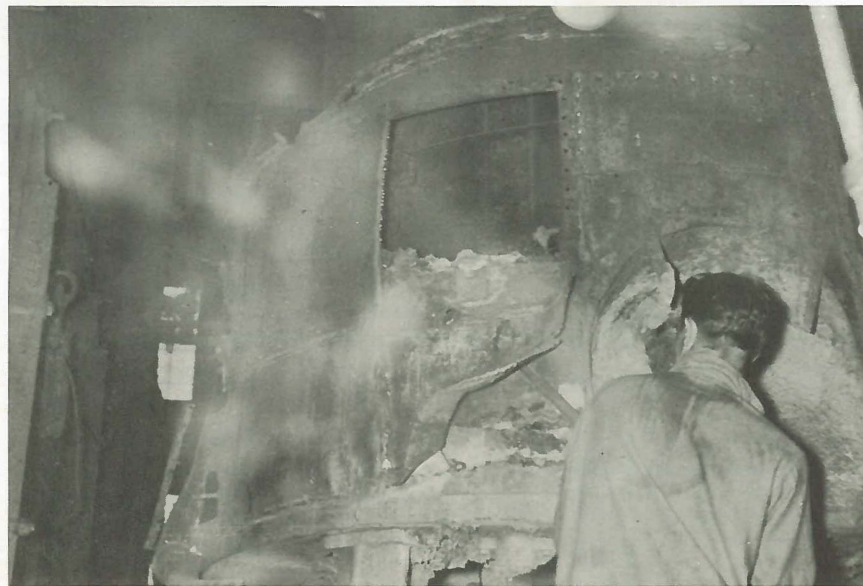
BOB MORRISON, using a small jack hammer, rips off a section of shell that cannot be reached with a torch.
