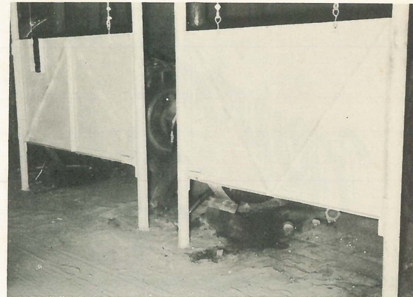
Shown here are the new tumbler guards that were recently installed in the Foundry Finish Dept.
