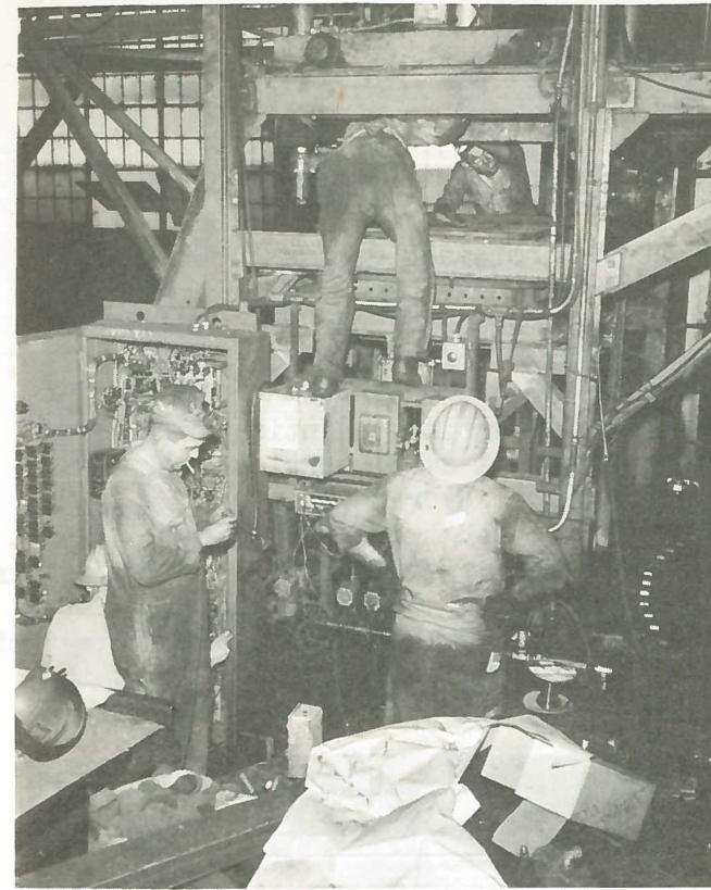
JAMES LAYTON, JOE SHORES, BILL HAYES and ALMOND NORRIS are shown re-wiring the flask placement station on the turntable operation and working on the flask stop in our Specials Foundry.
