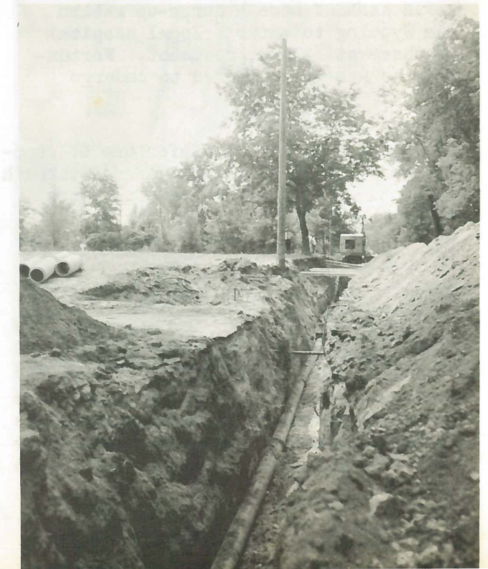
Below, the main in its new trench at new grade, ready for backfill, to complete the project.
