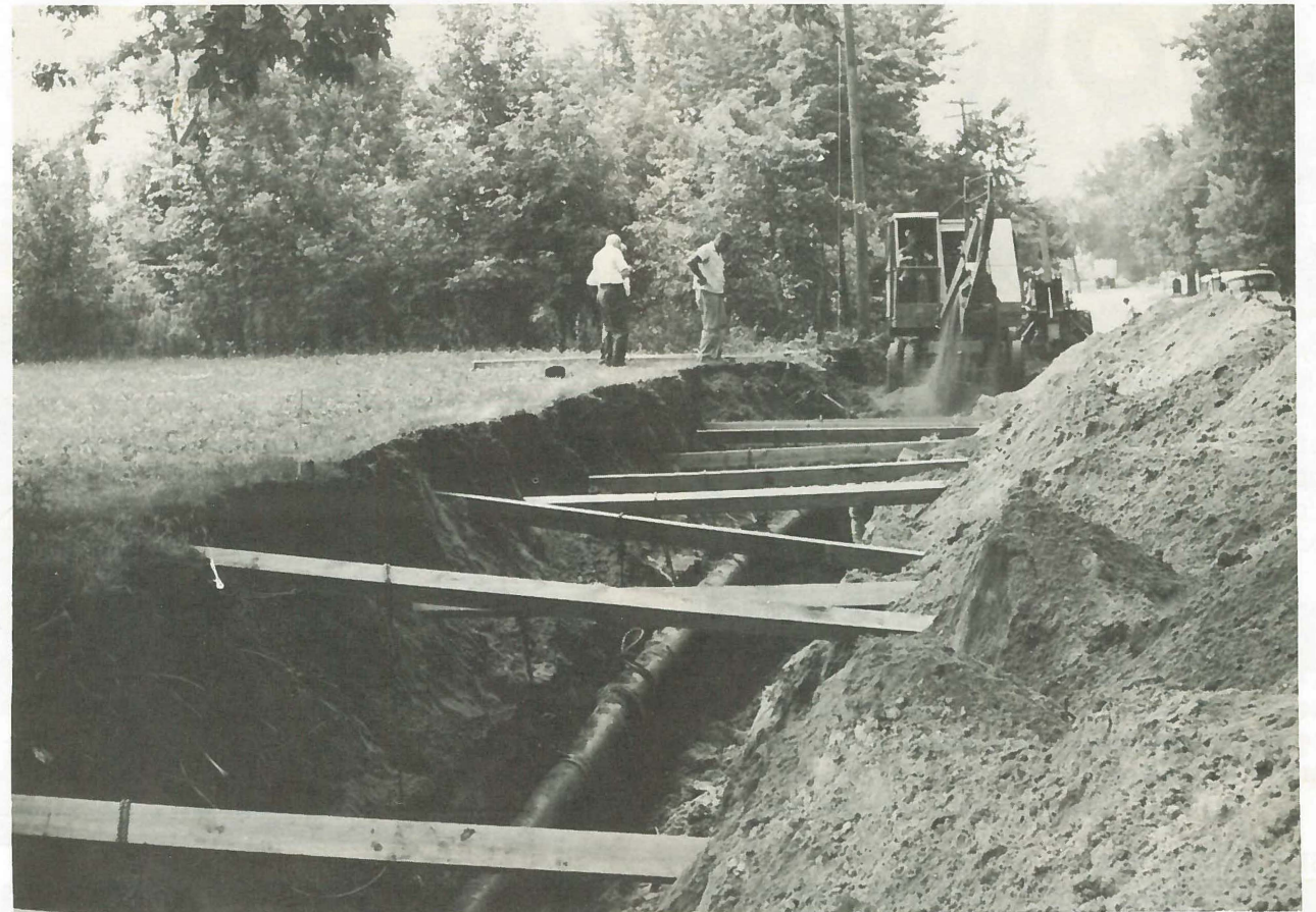
The method used to lower main is shown above, with the supporting lines tied to wooden beams across the open trench.
