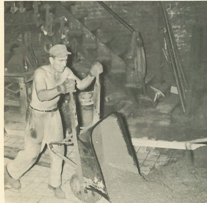
UBALDO BUONCAMPAGNI dumps a wheelbarrow load of concrete into a form that will become a base for our new sand machine.
