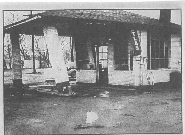
Photo courtesy of Luann (Huff) Fultz, North Canton This early-mid 1940s photo of the former Sohio Station, once located at the northwest corner of Pilling and State streets, Newcomerstown, shows damage to the structure after it was accidentally struck not once, but twice within the same week! The building was struck by a semi-truck/trailor outfit that was loaded with steel pipe the first time, then a different semi-truck struck the building the second time. The damage was estimated over $500 the first time. The manager of the station at that time was former Newcomerstown resident Lloyd "Pat" Huff.
