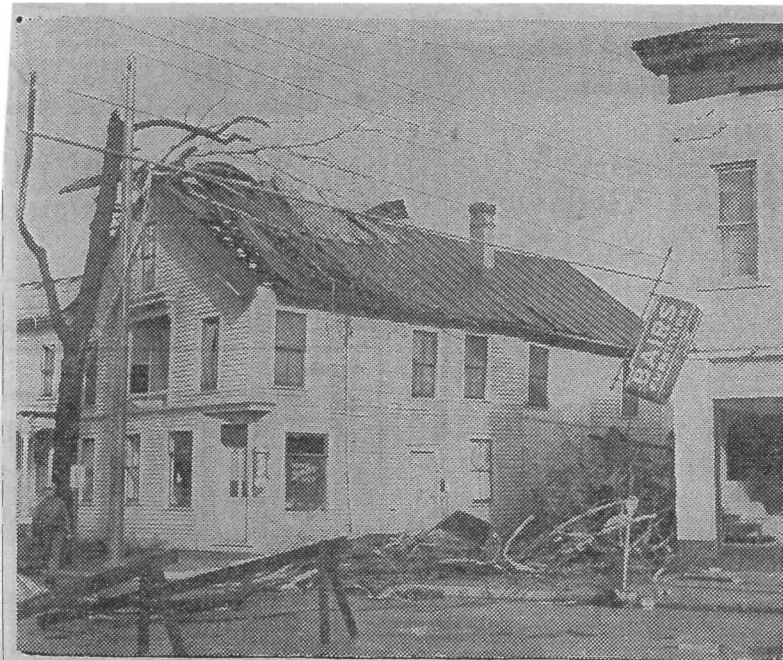
ROOF of the Main st. building owned by Mrs. Mellie Goudy was badly damaged in the Friday tornado. The second floor contained stored furniture. —Lenzo Photo
