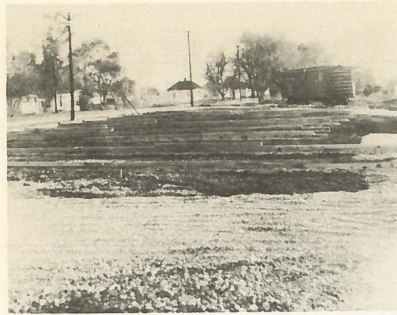
Looking south we see that our storage yard is ready for pipe.
