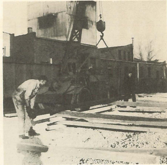
Charlie Long and Jim West roll a length of pipe on the storage ways.
