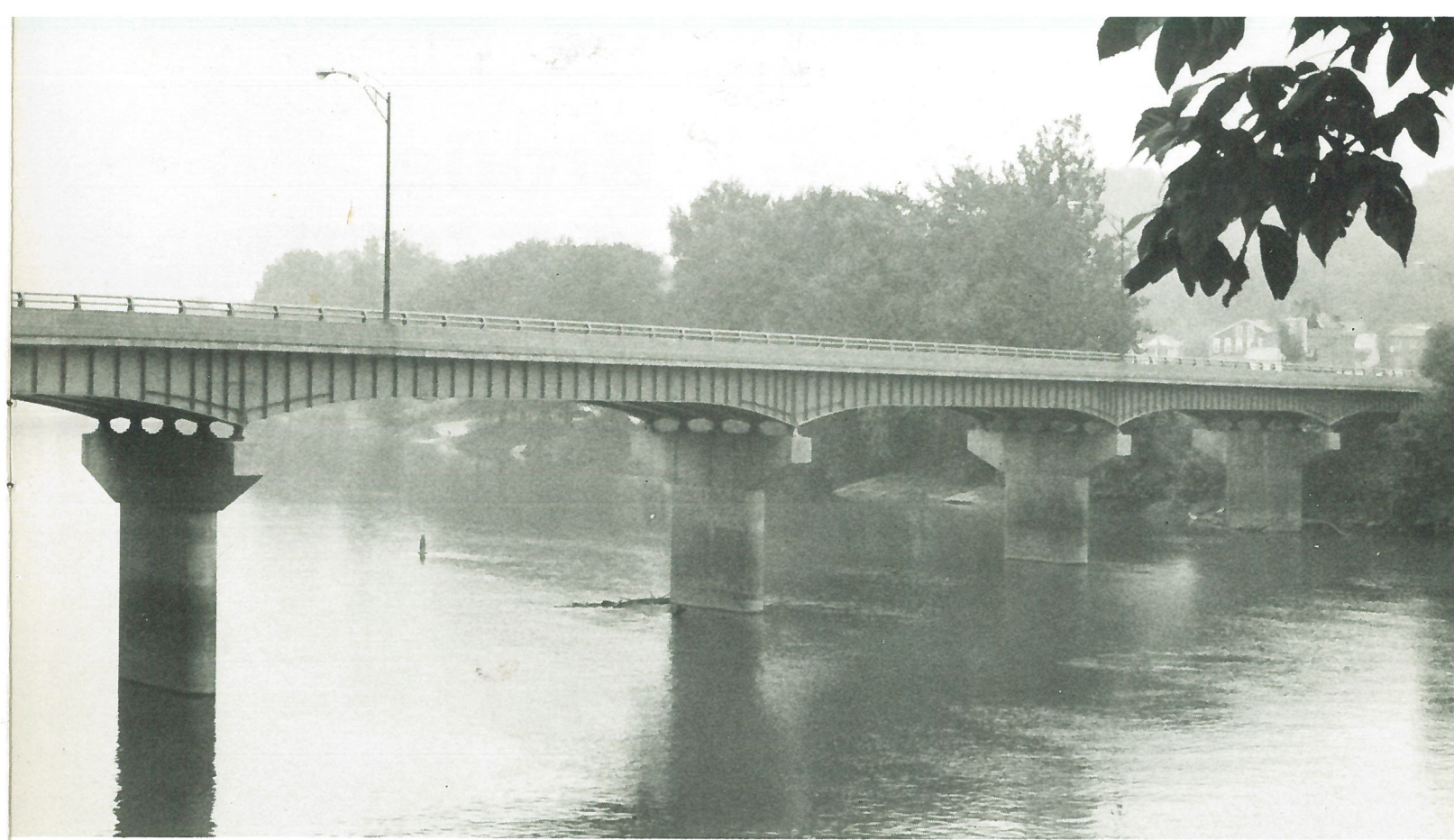
1963 — HIGHWAY BRIDGE — crosses both the Muskingum River and Wolf Creek on State Route 76 at Beverly, Ohio. Job for Ohio Department of Highways.
