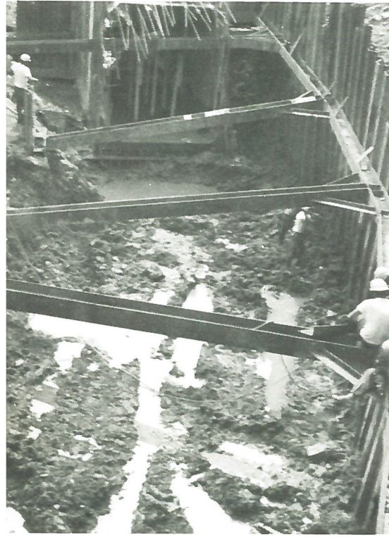
Struts are installed to brace the sheet piling retaining wall on this box culvert project at Baileysville, West Virginia — 1973.
