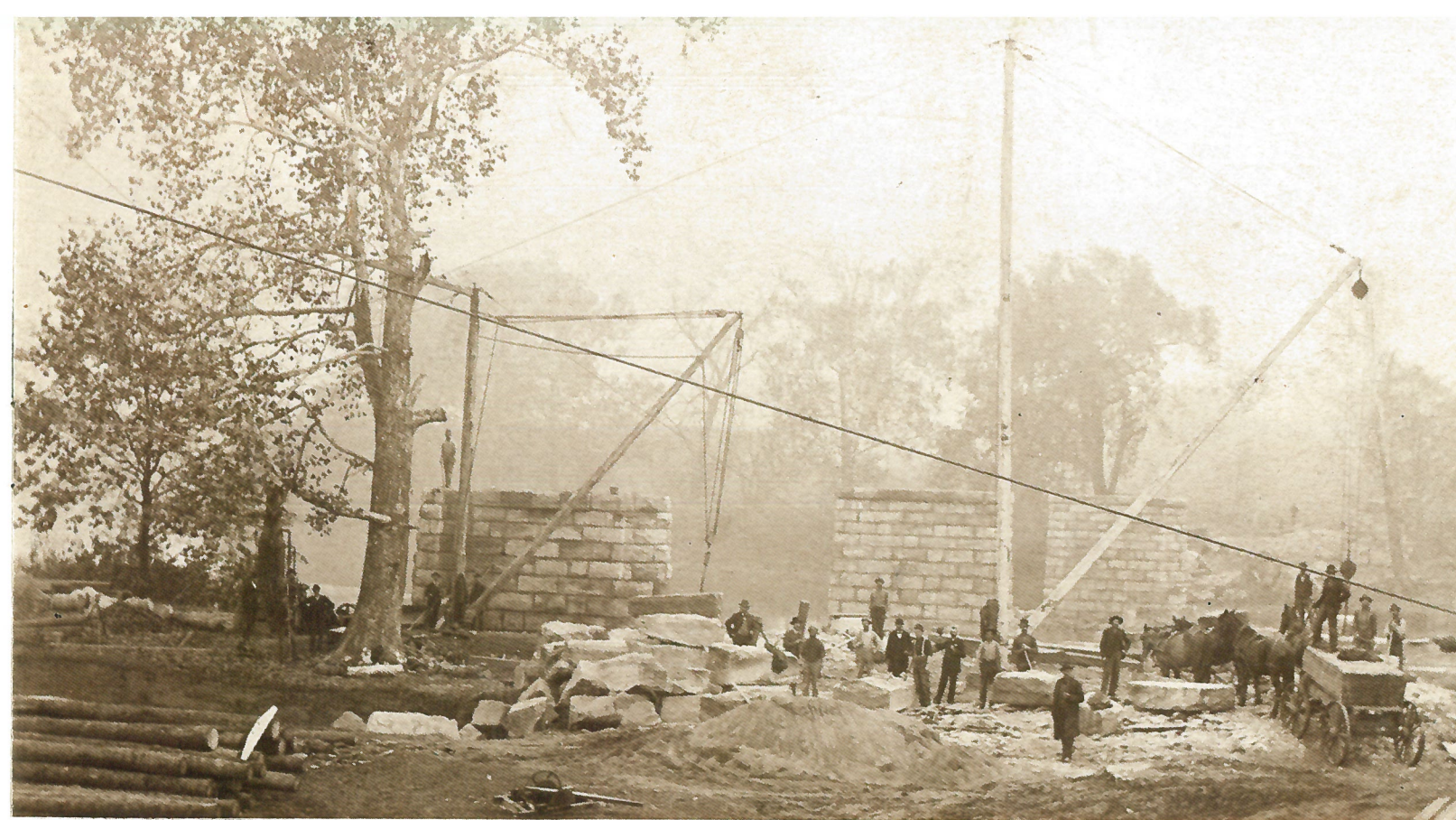
1891 Working on masonry piers for a bridge over the Tuscarawas and White Woman Rivers at Coshocton, Ohio. This job was for the Toledo, Walhonding Valley and Ohio Railroad.
