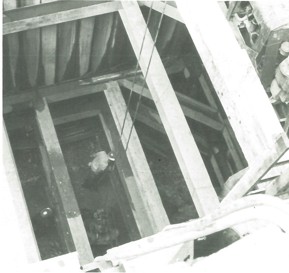
Excavating to grade for a pier footer on a state highway bridge project across the Muskingum River at Beverly, Ohio — 1963.
