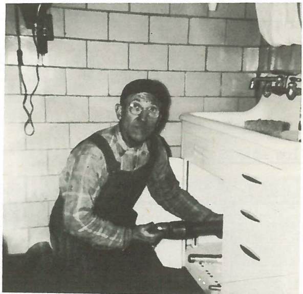
John Shaw , installing a cold water line for the First Aid Office.
